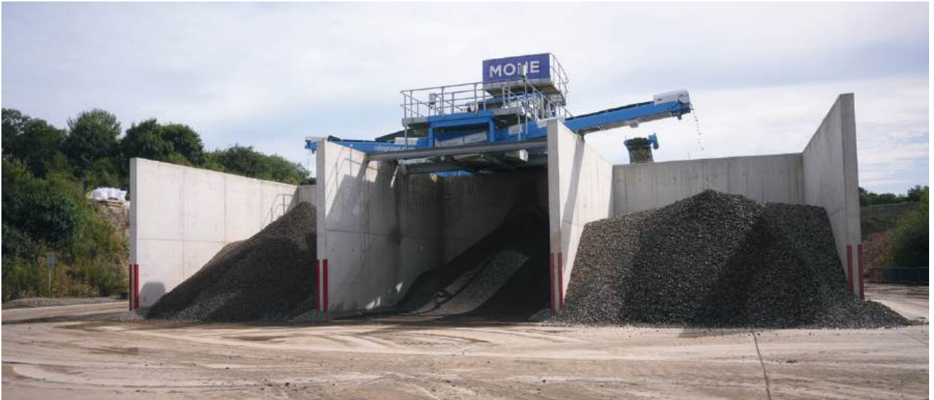
The CD&E waste-recycling plant allows Mone Bros to produce a range of high-quality recycled products
